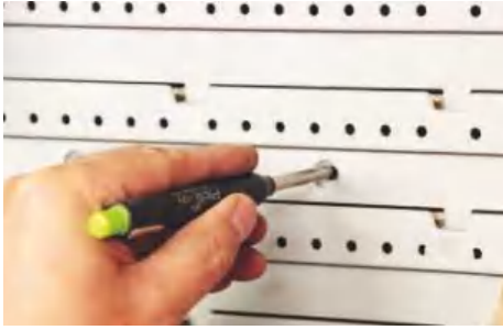
▲ The extending lead also proves useful for marking through fittings for hole positions
